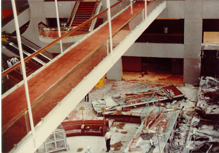
Figure 1-3. Aftermath of collapse. (Source: Lowery, L. (2007): Aftermath of Collapse. Retrieved October 15, 2007, from http://ethics.tamu.edu/ethics/hyatt/hyatt2.htm ).
