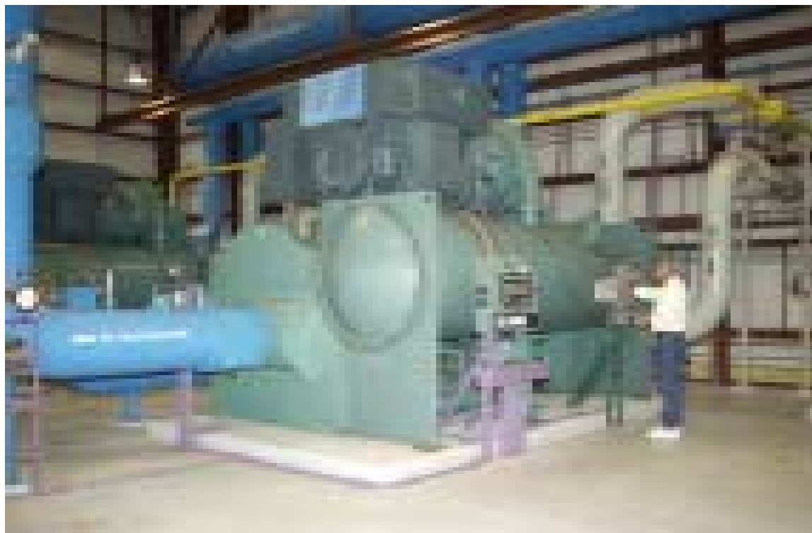
Left: This chiller unit circulates 4,500 Gallons per Minute (GPM) of chilled water.
