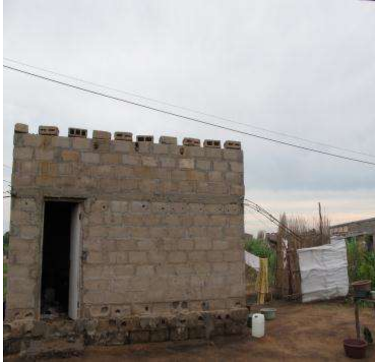
Figure 3-4. TAE Informant (Mario's) home in Matola constructed of cement received as an incentive for weapons exchange. Photograph by A. Schwartzott
