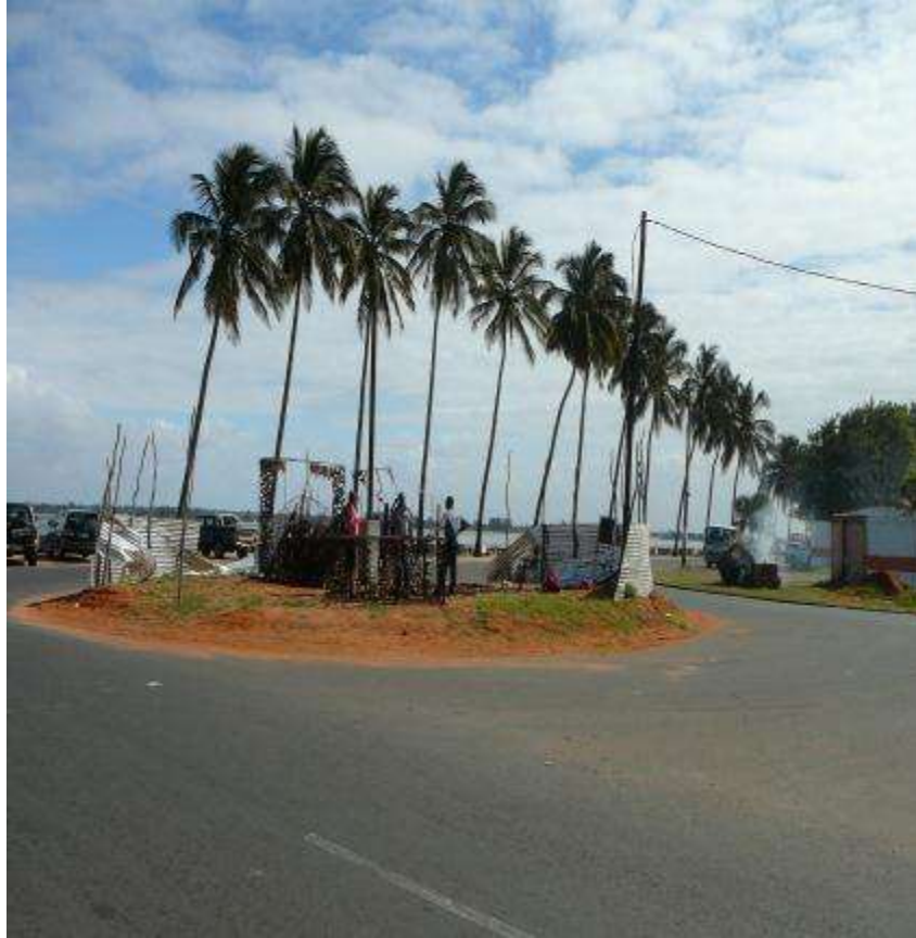
Figure 3-22. Kester, Site of intended monement, O Pombo da Paz/The Dove of Peace , in construction, August 2009. Photograph by A. Schwartzott
