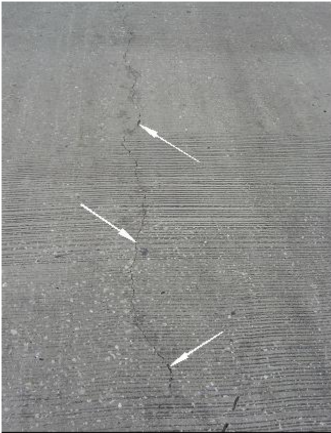
Figure 3. Reflective crack on topping of Mill Creek Bridge
