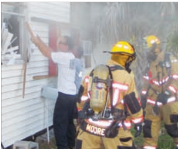
Rescue teams cut a hole in the side of the building to allow smoke to escape
