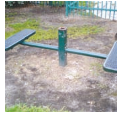
Safety alert: The city needs to attend to this hazard immediately.
