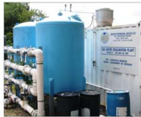
Desalination Plant, Carriacou, Grenada
