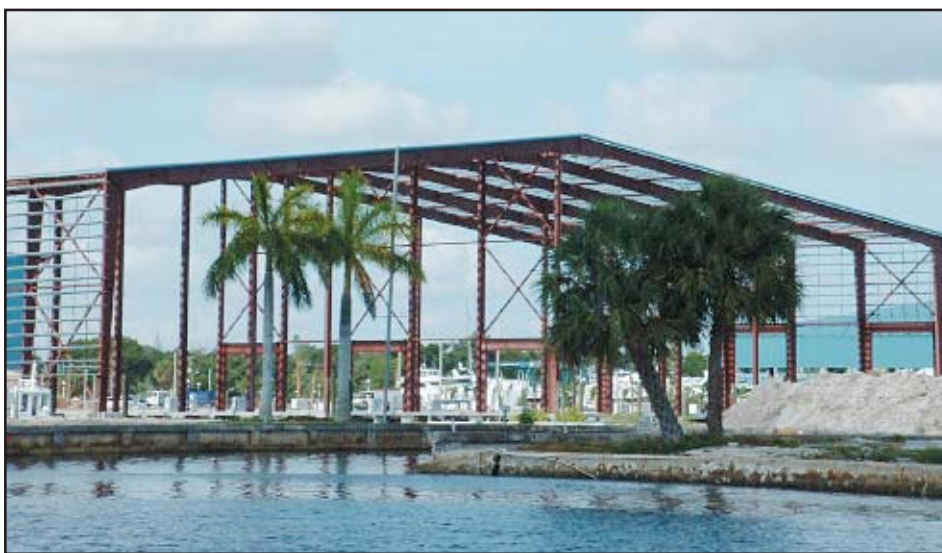
Lauderdale Marine Center's attempts to build a new boat shed are being protested by neighborhood residents who say the project is intrusive.
