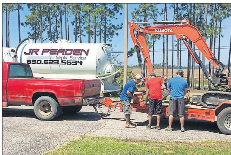
JR Peaden Septic Service replaced My Father's Arrows' entire commercial septic system just for the cost of materials, which saved MFA about $10,000 after discovering the unexpected need to replace it. "Their donation has allowed us to create more licensed beds in our county," MFA Executive Director Sarah Ellis said. [SPECIAL TO THE PRESS GAZETTE]
