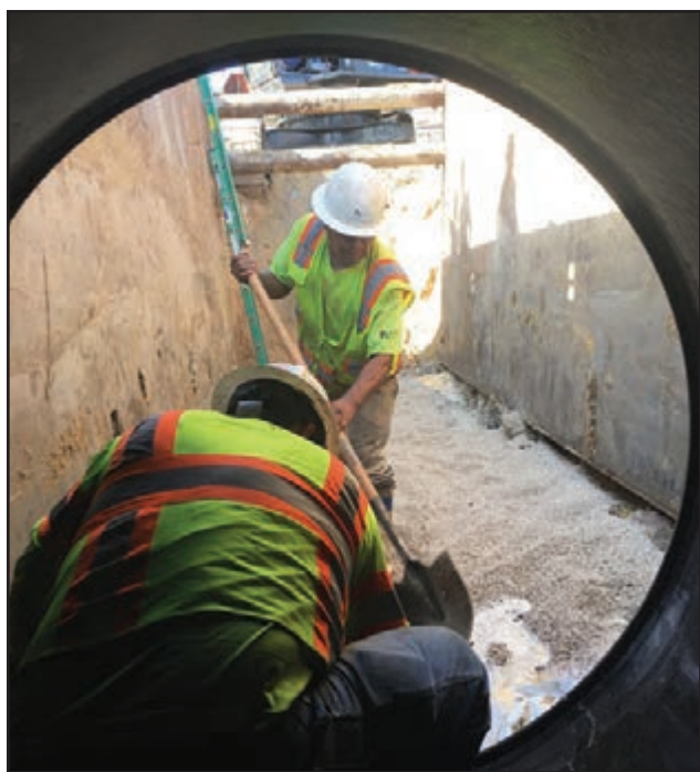
Two construction workers work from a trench box to safely install pipe.
