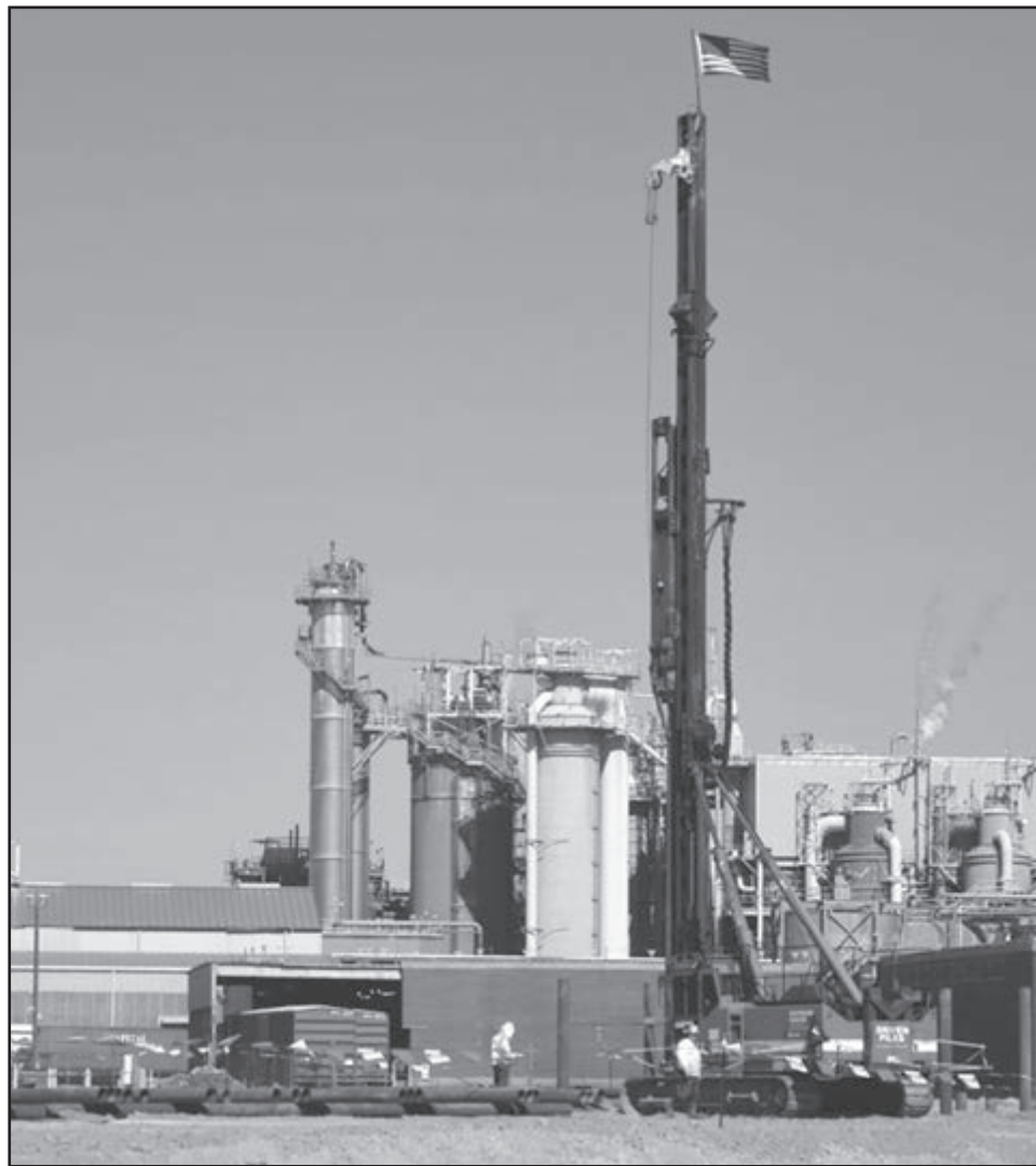
With the former Human Resources building demolished, site preparations continued in February and March for construction of additional warehouse space.
