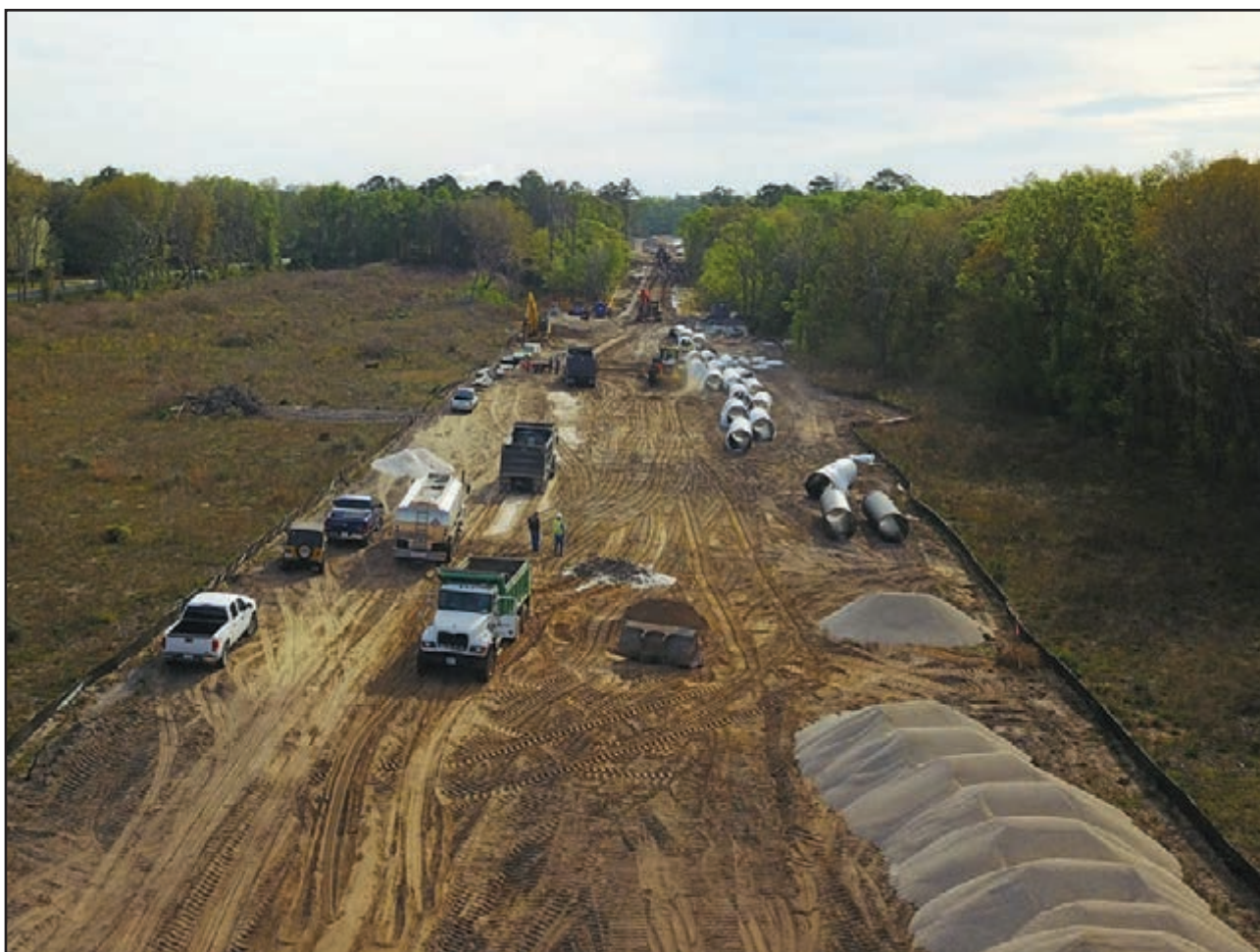
Construction of the 15.3-mile pipeline began in December 2018 and will continue for an estimated 14 months until March 2020. In February, the project team adjusted the construction schedule and proceeded with construction activity along Carlton Cemetery Road (shown above).
