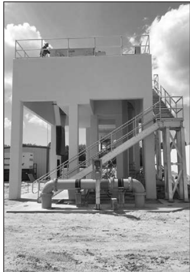
The City of Perry is nearing the completion of construction of the city's newest and largest wastewater treatment plant, a $15 million project. "Industry cannot come here if the infrastructure of the city can't support it," City Manager Taylor Brown said.
