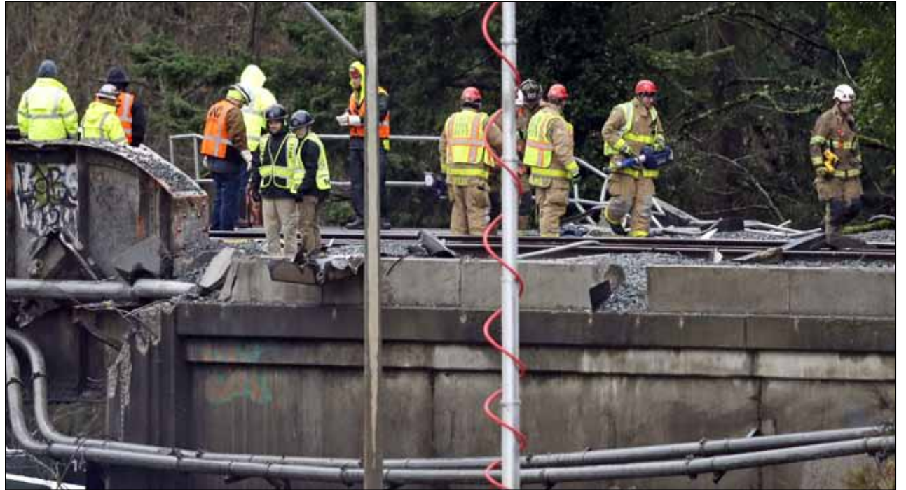
Workers stand atop a damaged railroad bridge at the scene of an Amtrak train crash onto Interstate 5 a day earlier Tuesday, Dec. 19, 2017, in DuPont, Wash.
