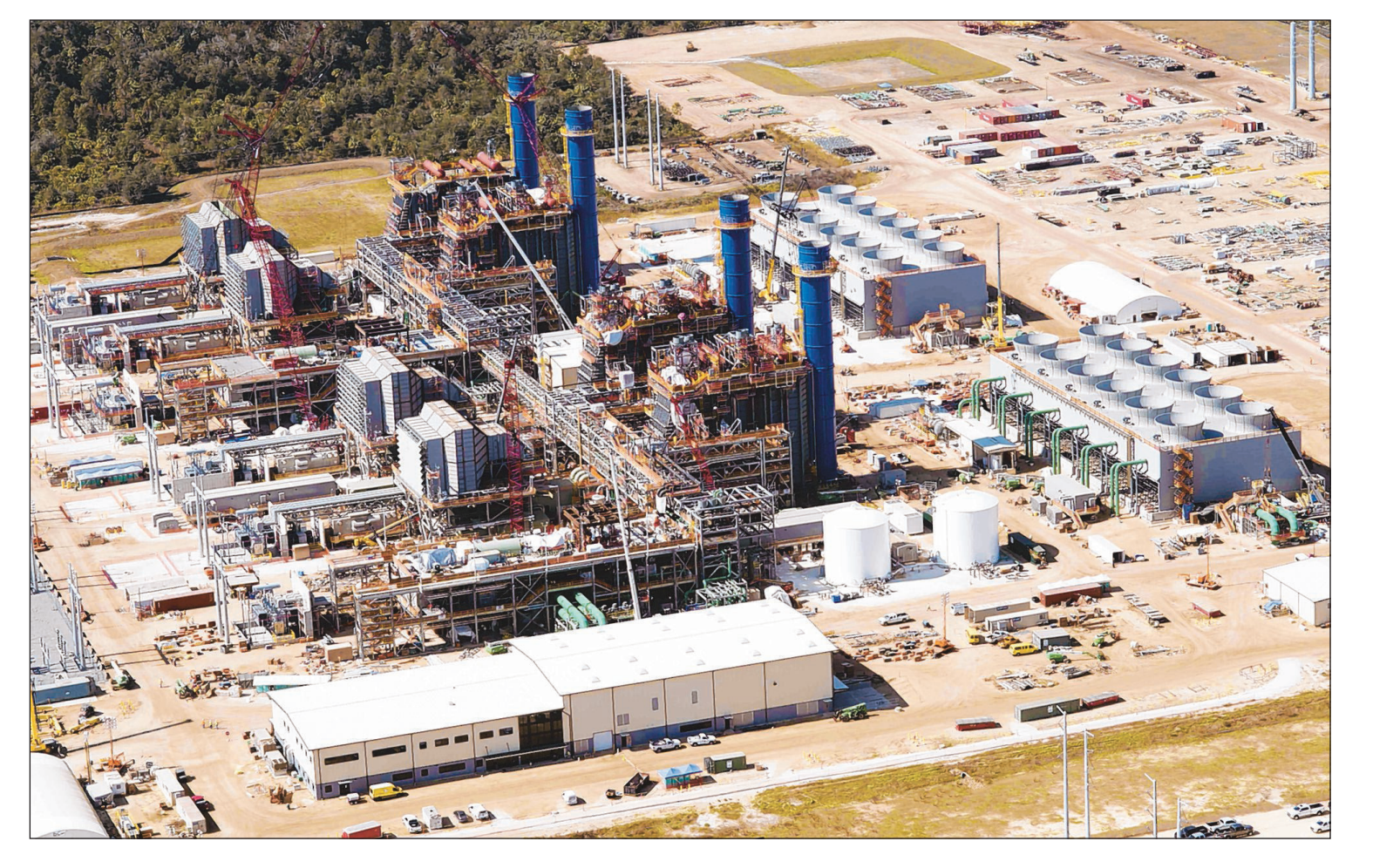
This aerial photo shows the Duke Energy gas plant under construction in November 2017. Special to the Chronicle
