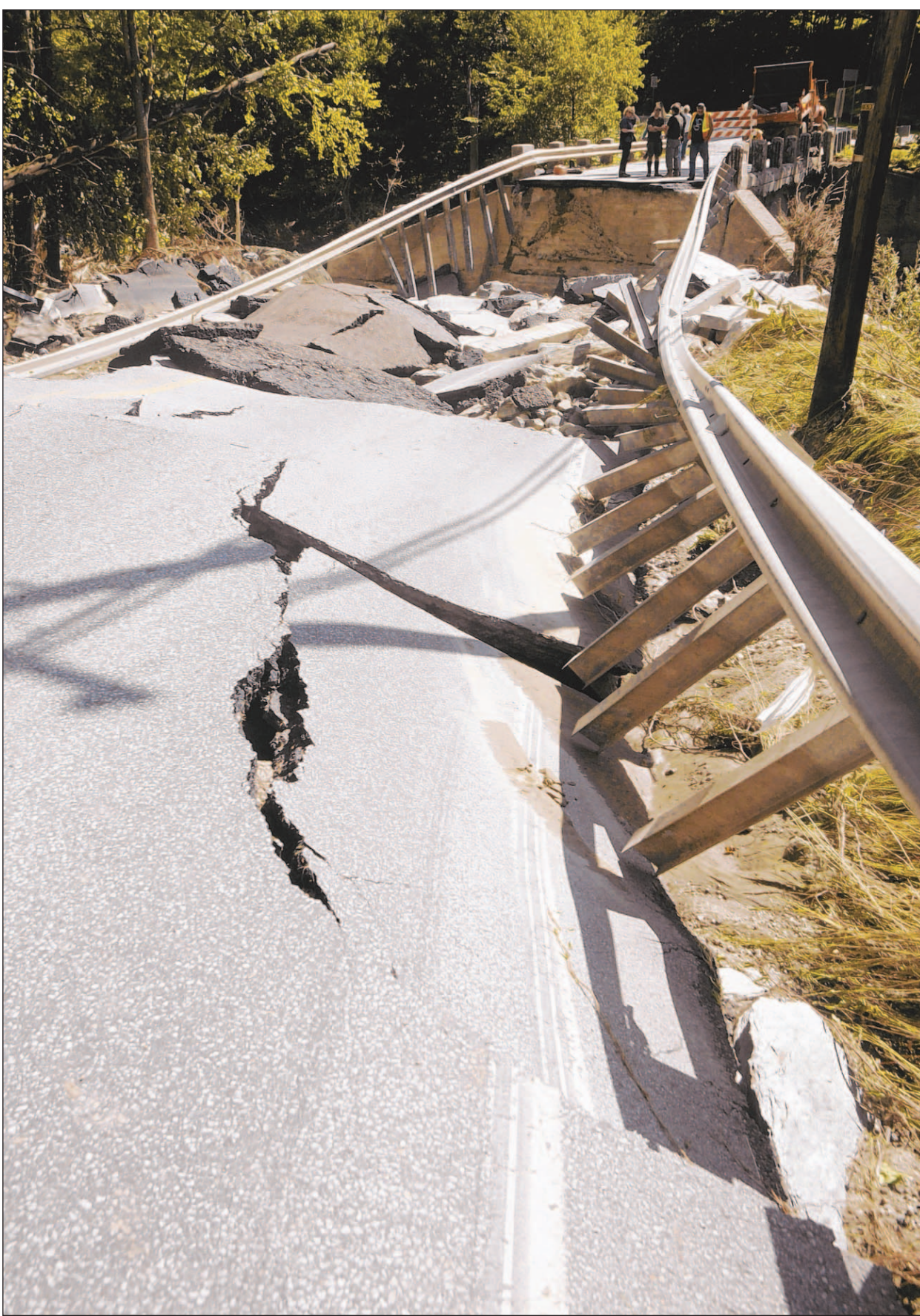
People view the washed-out roadway of Route 100B on Monday in Moretown, Vt. The road was destroyed by the rain-swollen Mad River when Tropical Storm Irene passed through on Sunday.
