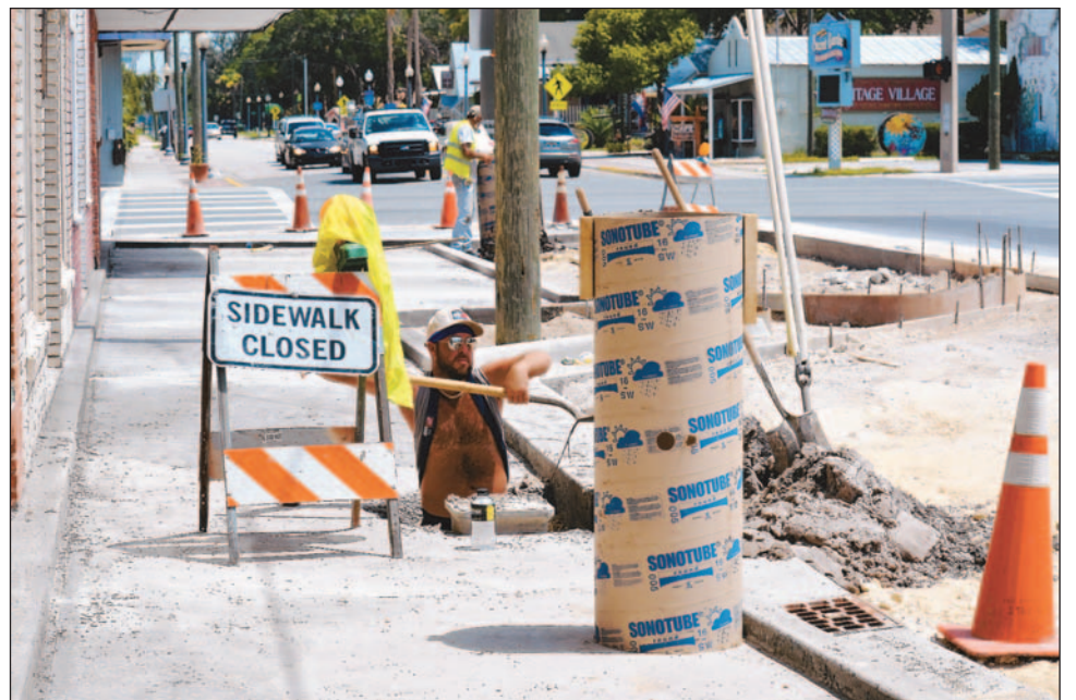
RIC BUSH/Special to the Chronicle Matt Cousteau works below ground last week on the new sidewalk going in on Citrus Avenue in Crystal River.
