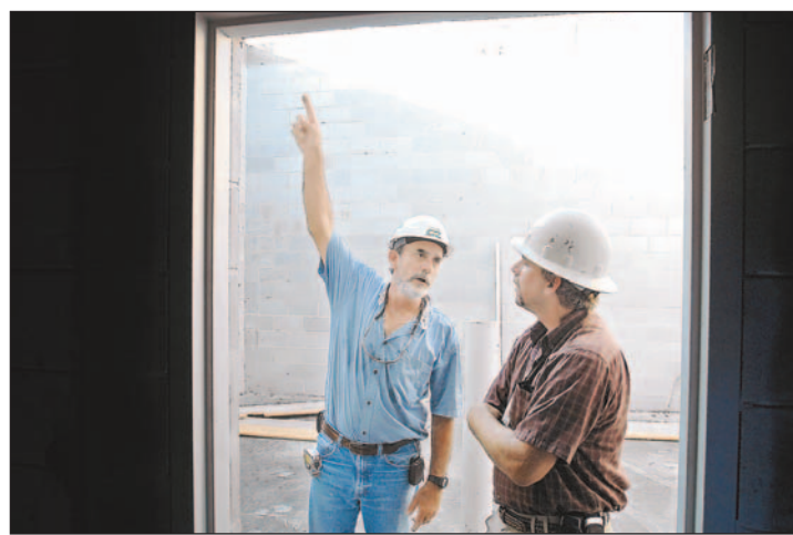
Chuck Durden, superintendent at the CRPS construction site, left, confers with Eric Stokes, the project manager who works for the school district.
