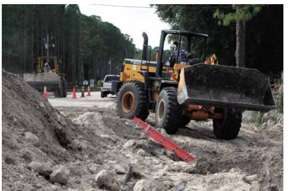
A bulldozer clears dirt in the ditch near Chiefland Elementary School as part of a sewer improvement project.
