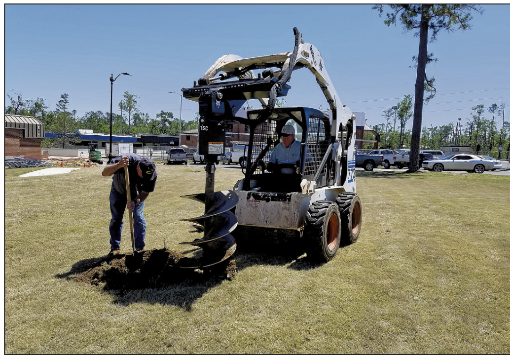
Chipola College maintenance man Ben White and Chipola's Facilities Director Richard Rehberg, operating auger, prepare the planting space for a white oak tree with historic origins.
