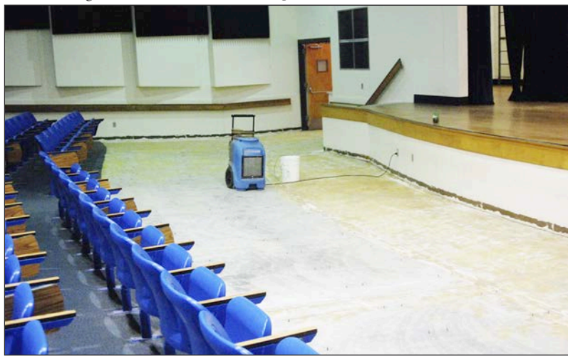
District school officials are eyeing a costly fix to flooding inside the Hardee Senior High School auditorium. In this photo taken Sept. 18, rows of chairs were removed to allow crews to clear away flood-damaged flooring in the auditorium.
