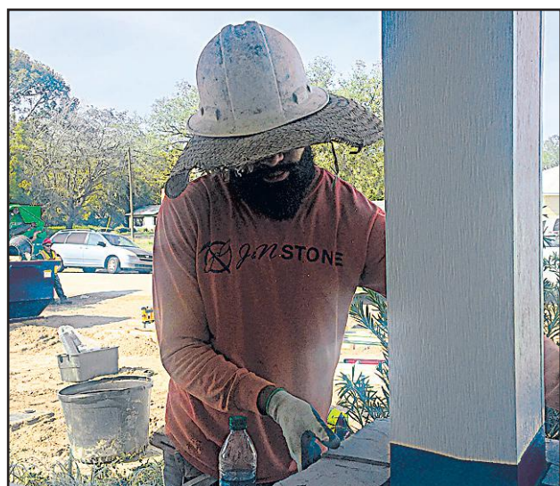
A volunteer from a professional construction company lays down stone around the column of a house during Builders Blitz at Arbor Bend.
