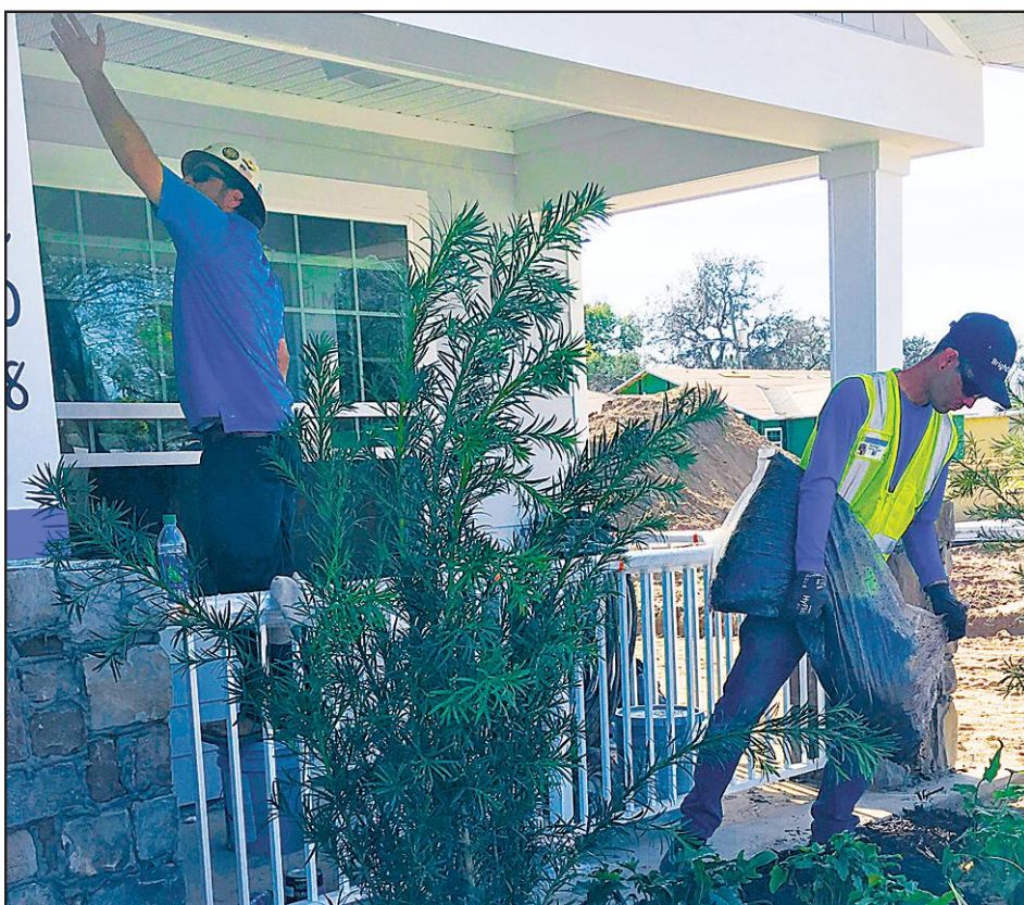
Volunteers from four professional builders construct four houses in five straight days during Habitat for Humanity's Builders Blitz, doing various jobs ranging from landscaping to infrastructure work.
