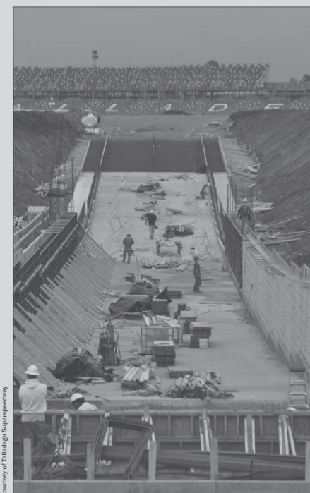
Crews work on the new, large tunnel that will provide access to the Talladega infield through Turn Three.
