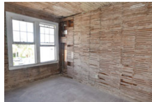
Inside one of the many rooms on the upper floors of the old hotel that will be renovated into boutique-style apartments.
