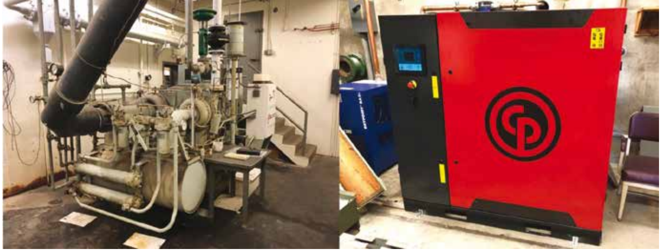
The old 500 kW compressor (left) was replaced with a 55-kW compressor (right).
