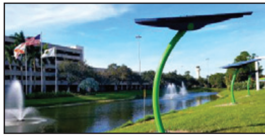
Florida Power & Light's solar trees at Palm Beach International Airport. The partnership between the utility and the airport comes from FPL's SolarNow program.
