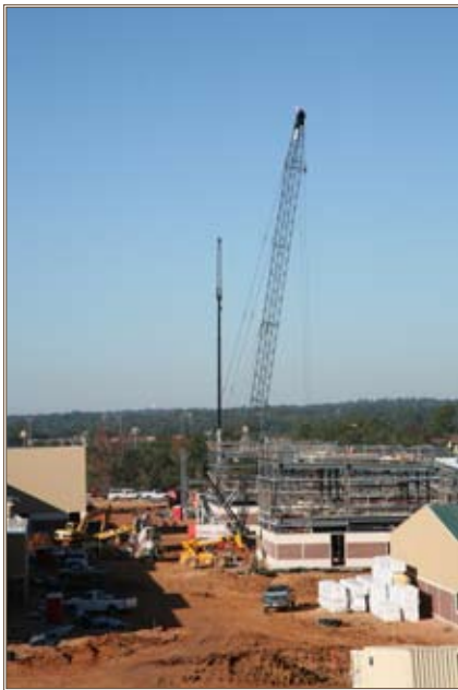
Barracks are under construction at Fort Benning, Ga. Photo by F.T. Eyre, Headquarters, U.S. Army Corps of Engineers
