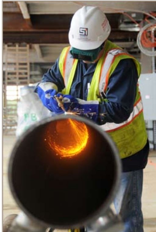
Steamfitter James Chandler cuts a steel chillwater pipe at the site of the Fort Belvoir (Va.) Community Hospital, a BRAC project that will provide a 120-bed, state-of-the-art facility. Photo by Marc Barnes, Belvoir Integration Office, U.S. Army Corps of Engineers
