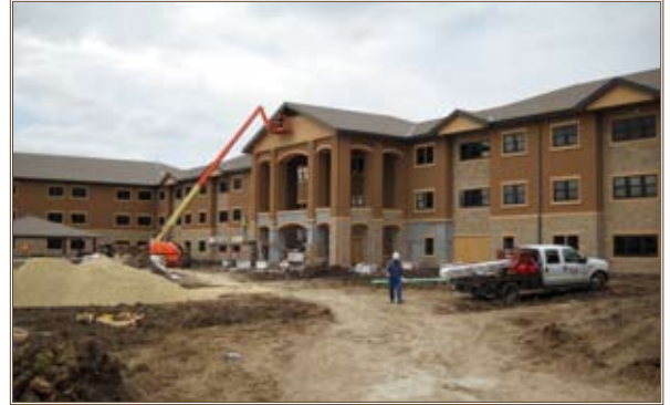
Construction is under way on a Warriors In Transition campus at Fort Riley, Kansas. Photo by Robert G. Dye, Kansas City District, U.S. Army Corps of Engineers
