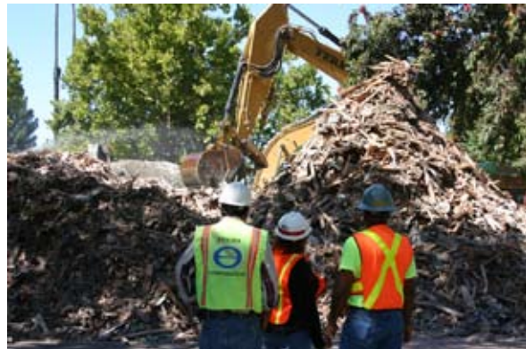
Gregorio Pena (left), Ferma Corp., Mindy Shelton, Huntsville Center, and Milton Dozier, Bhate Associates, watch a backhoe crunch debris at Moffett Field. Photo by Debra Valine
