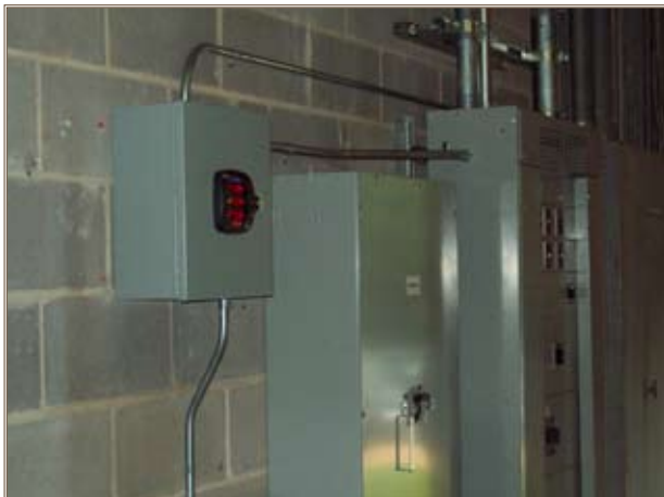
These advanced meters, part of the Army Metering Program, capture electricity and natural gas consumption at Redstone Arsenal, Ala. Photo by Patrick Holmes, Johnston Controls Huntsville
