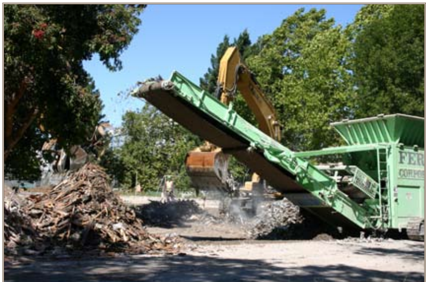
A crusher grinds building debris so it can be recycled for other uses as part of the FRP. Photo by Debra Valine
