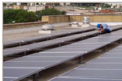
A worker installs photovoltaic solar panels on Bldg. 1350 at Fort Sam Houston, Texas. Photos courtesy of USACE Public Affairs
