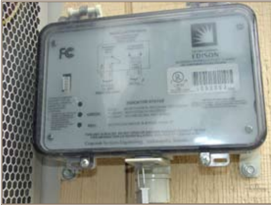
Cycling devices on air conditioners in housing units allow Fort Irwin to receive credits on summer electric bills in exchange for permitting the utility to periodically turn off the air conditioners. Photo by Hossam Kassab
