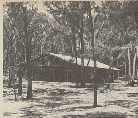
RAINBOW SPRINGS will soon feature a Quarter Horse attraction. Shown here is the completely modern horse barn under construction at the Florida attraction. Regular Quarter Horse performances will be held on a daily basis in the adjacent arena, also under construction.
