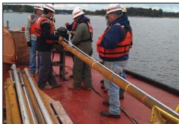
Norfolk District personnel work with equipment borrowed from New York District as they take coring samples in Virginia. (Photo by Mike Folcik, New York District Operations Division)
