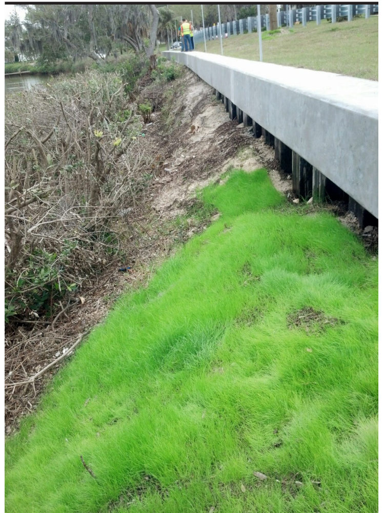
Now that the project is completed, shorelines and adjacent roadways are protected. The evacuation area and homes are protected from the bayous. (Photo courtesy of Jim Suggs)
