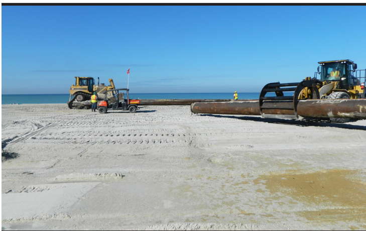
Corps contractors Great Lakes Dredge and Dock move pipe along an Anna Maria Island beach in February. The offshore dredge vessel pumps sand through miles of pipes onto the beach. Cages at the opening of the pipeline capture debris such as shells, rocks and other objects to prevent their placement on the beach. (Photo by Brian Austin)
