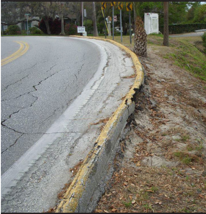
Prior to the Whitcomb and Kreamer Bayous Hurricane and Storm Damage Reduction Project, the banks experienced erosion that threatened city- and county-maintained roadways. (Photo courtesy of Jim Suggs)
