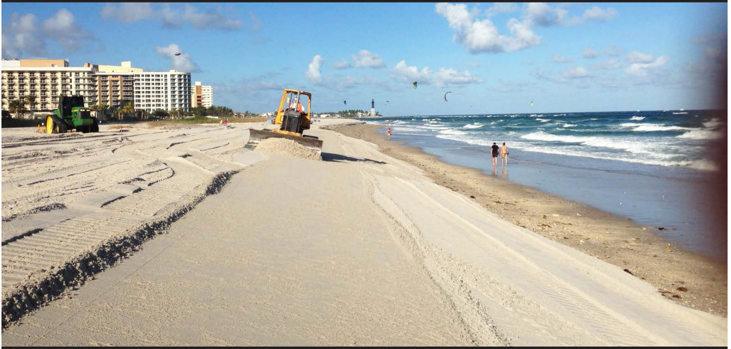
Workers flatten delivered sand on a Broward County beach so it fills an engineer-designed template, which includes the sand placement's height and width along the beach. (Photo courtesy of Eastman Aggregate Enterprises)
