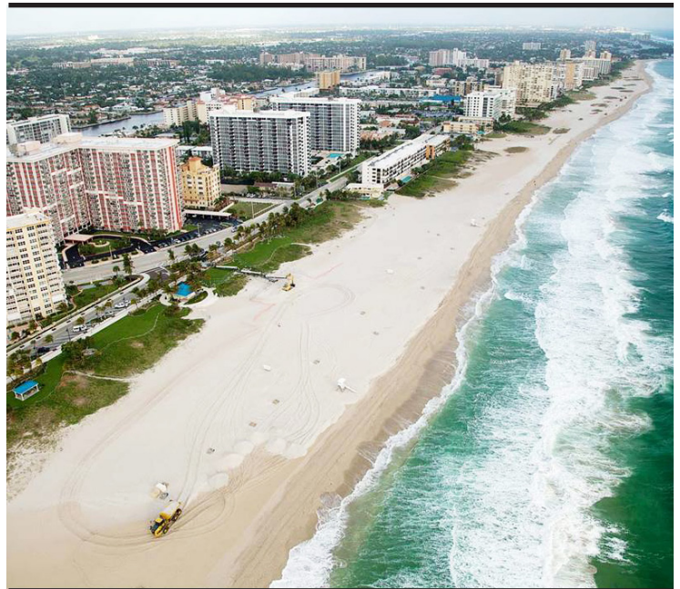
Workers place a layer of sand that renourishes beach-eroded areas along the Broward County shoreline. The district is restoring more than 38 miles of federal shore projects in Florida that were eroded by storm-induced waves in 2012. (Photo courtesy of Eastman Aggregate Enterprises)
