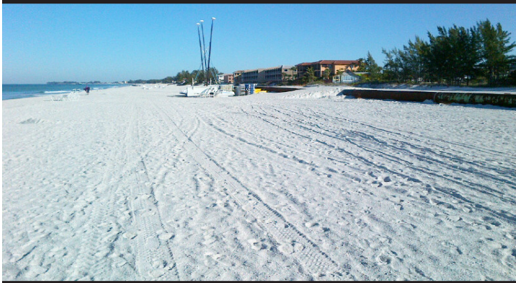
A near-completed portion of beach renourishment on Anna Maria Island. (Photo by Brian Austin)
