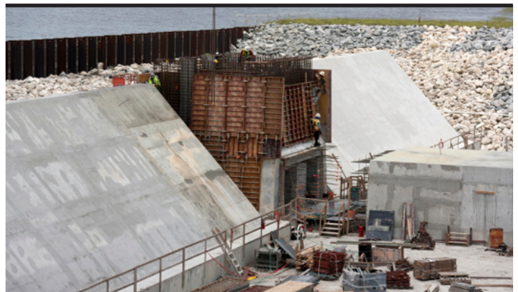
Rehabilitation work continues at Herbert Hoover Dike, with the replacement of more than 30 water control structures around the lake, similar to the Culvert 11 site pictured above. Jacksonville District plans to continue work to replace these structures through 2018. (USACE file photo)
