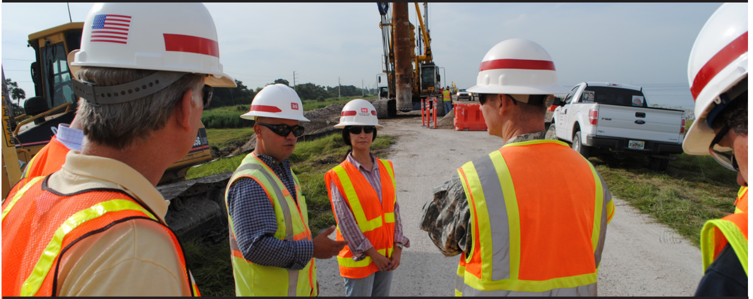
Col. Alan Dodd (right), district commander, is briefed by Mario Fuquene and Eva Porras on cutoff wall installation near Canal Point during a visit to Herbert Hoover Dike in October. Rehabilitation work at the dike was recently named the Outstanding Project of the Year by the American Society of Civil Engineers, Palm Beach Branch. (Photo by John Campbell)
