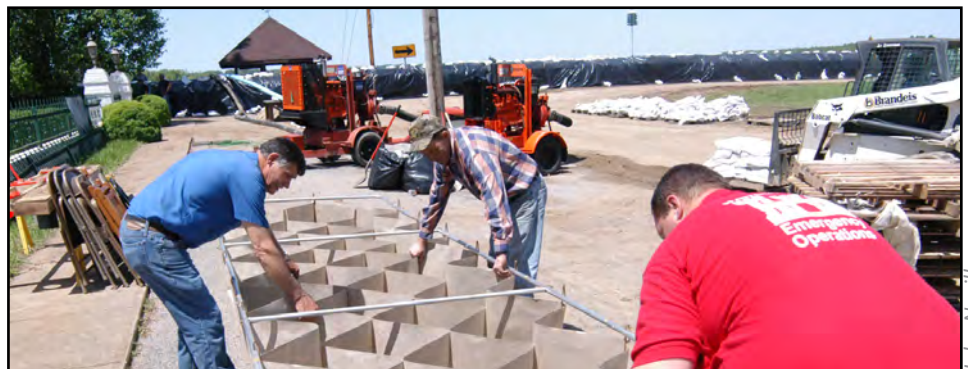
Louisville District geotechnical engineer Steven Shifflett and two locals demonstrate the assembly of The Typar® geocells in Smithland, Ky. The Louisville District flood fight team and the rest of the district’s emergency operations team decided to use the Typar® geocells instead of sandbags.
