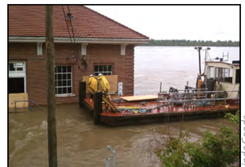
The crew at Lock and Dam 53 on the Ohio River covers the power house windows with plywood to keep drift from breaking them as the river level increased during the spring floods.
