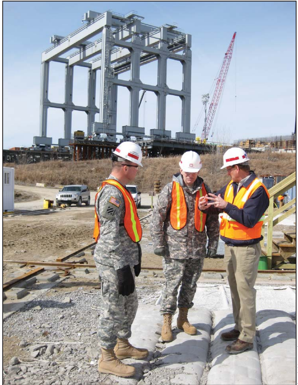
Rick Schipp (right) leads Maj. Gen. William Grisoli (center) and Col. Keith Landry on a tour of the Olmsted construction site.
