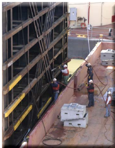
The Louisville Repair Station crew works to clean the miter gate leaf at Markland.
