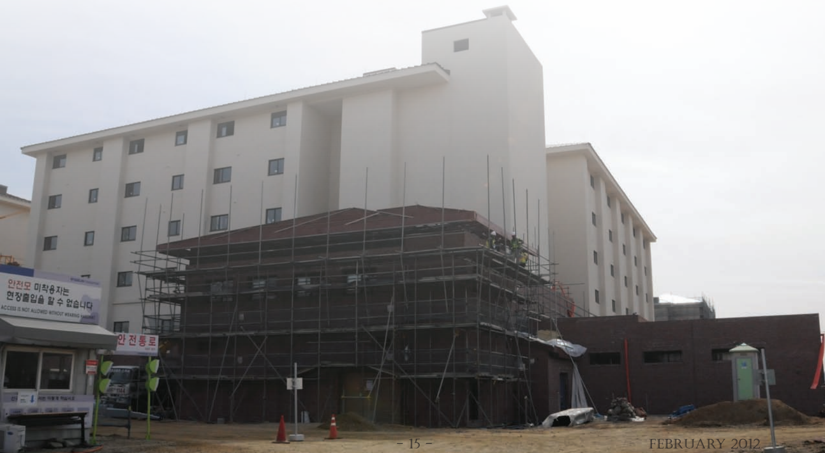
Buid-to-lease Senior Leaders’ Quarters under construction at U.S. Army Garrison Humphreys. (Photo by Patrick Bray)
