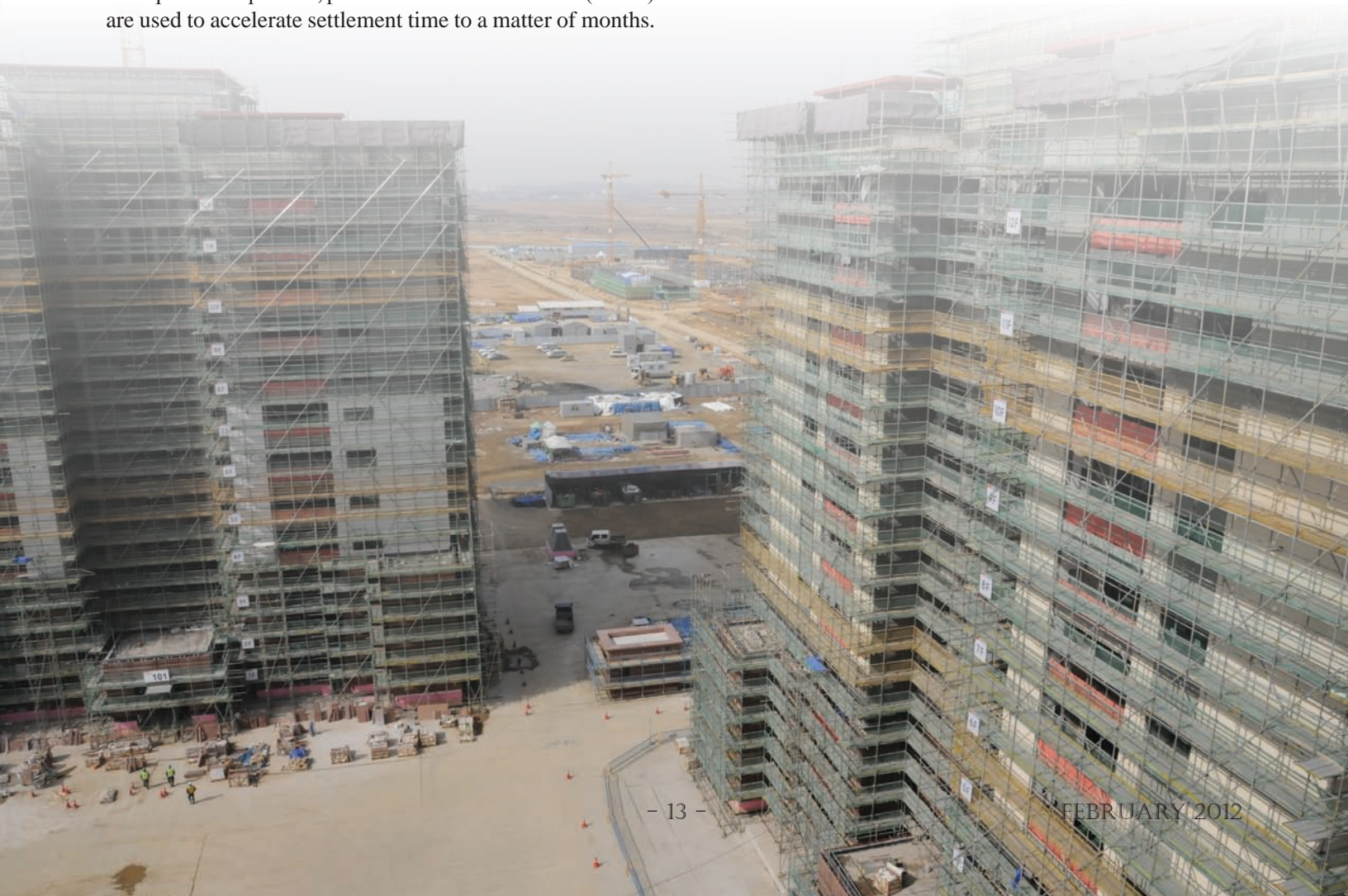
Army Family Housing Towers under construction at U.S. Army Garrison Humphreys. (Photo by Patrick Bray)
