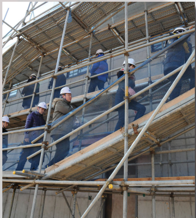
Engineers from the Korean Ministry of National Defense climb scaffolding to view rooftop construction on a project at USAG Humphreys during the MND Exchange Program Feb. 16. (Photo by Patrick Bray)
