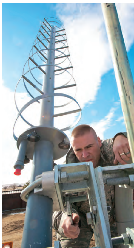
BELOW: A transmission system radio maintainer mounts a helical antenna to an AM-1 to send and retrieve information via satellite. Photo by Airman 1st Class Zachary Hada, U.S. Air Force.
