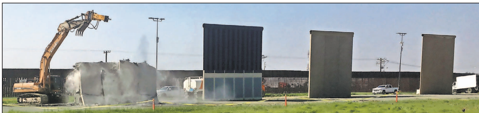
The government on Wednesday began demolishing eight prototypes of Donald Trump's prized border wall that instantly became powerful symbols of his presidency when they were built nine months after he took office.
