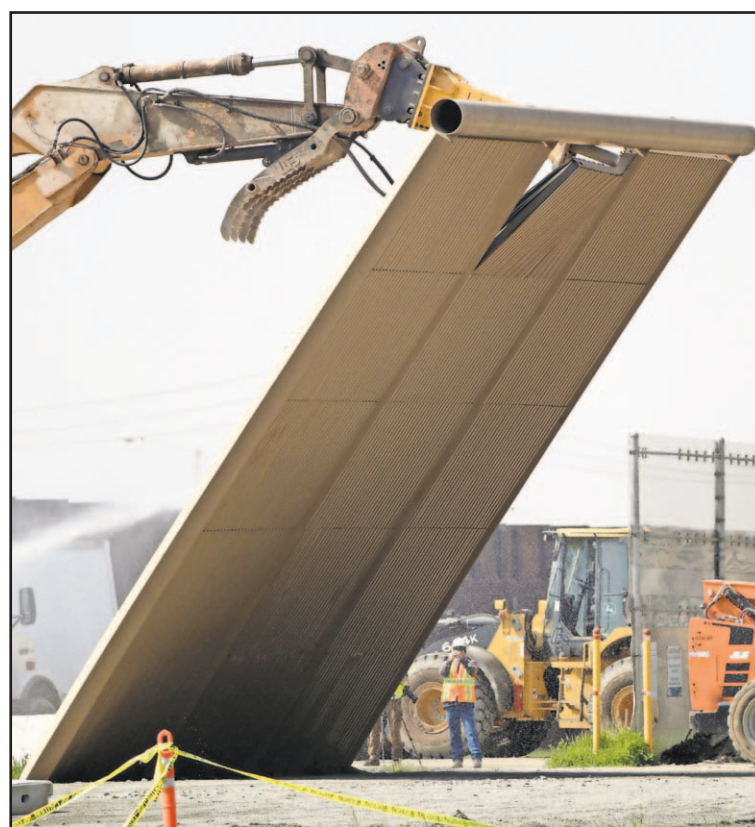
A border wall prototype falls during demolition at the border between Tijuana, Mexico, and San Diego, Wednesday.
