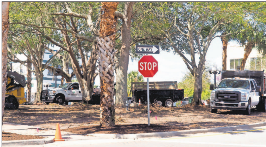
The Sebring CRA authorized work to begin on a downtown beautification project, but the agency did get bids on the work. This picture shows work being completed on Circle Park.
