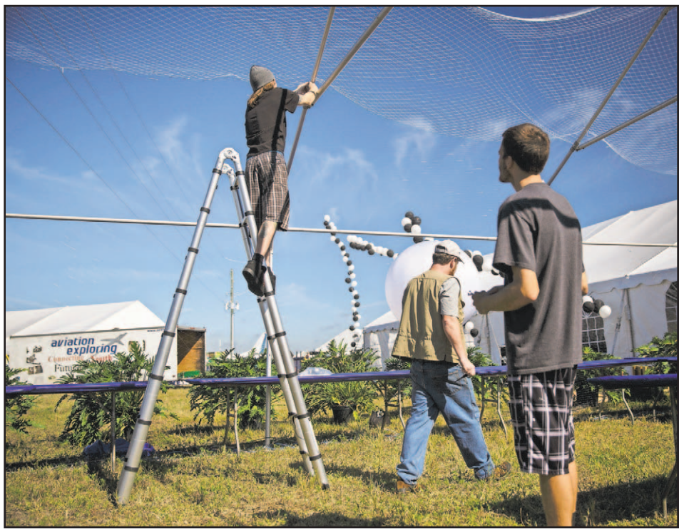
Workers install a "drone netting" to enclose the spectator area for the series of drone races at last year's U.S. Sport Aviation Expo.
