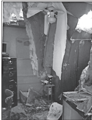
Part of the roof of The Church of God of Prophecy was ripped off during Hurricane Irma.
