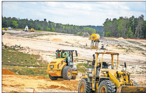
Crews work on the Suncoast Parkway in Hernando County where it crosses U.S. 98 on April 4. Environmental advocates worry that legislation being pushed by Florida Senate President Bill Galvano to build or expand three toll roads — including the Suncoast Parkway — will lead to suburban sprawl that will exacerbate Florida's environmental problems. [ALAN YOUNGBLOOD/GATEHOUSE MEDIA]
