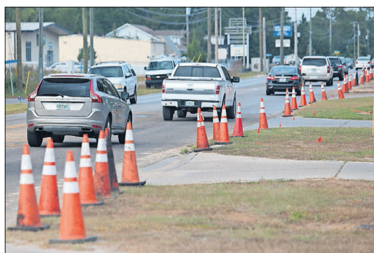
Cones are placed along Jenks Avenue north of 23rd Street in preparation for the widening project on Oct. 26, 2016. [NEWS HERALD FILE PHOTO]
