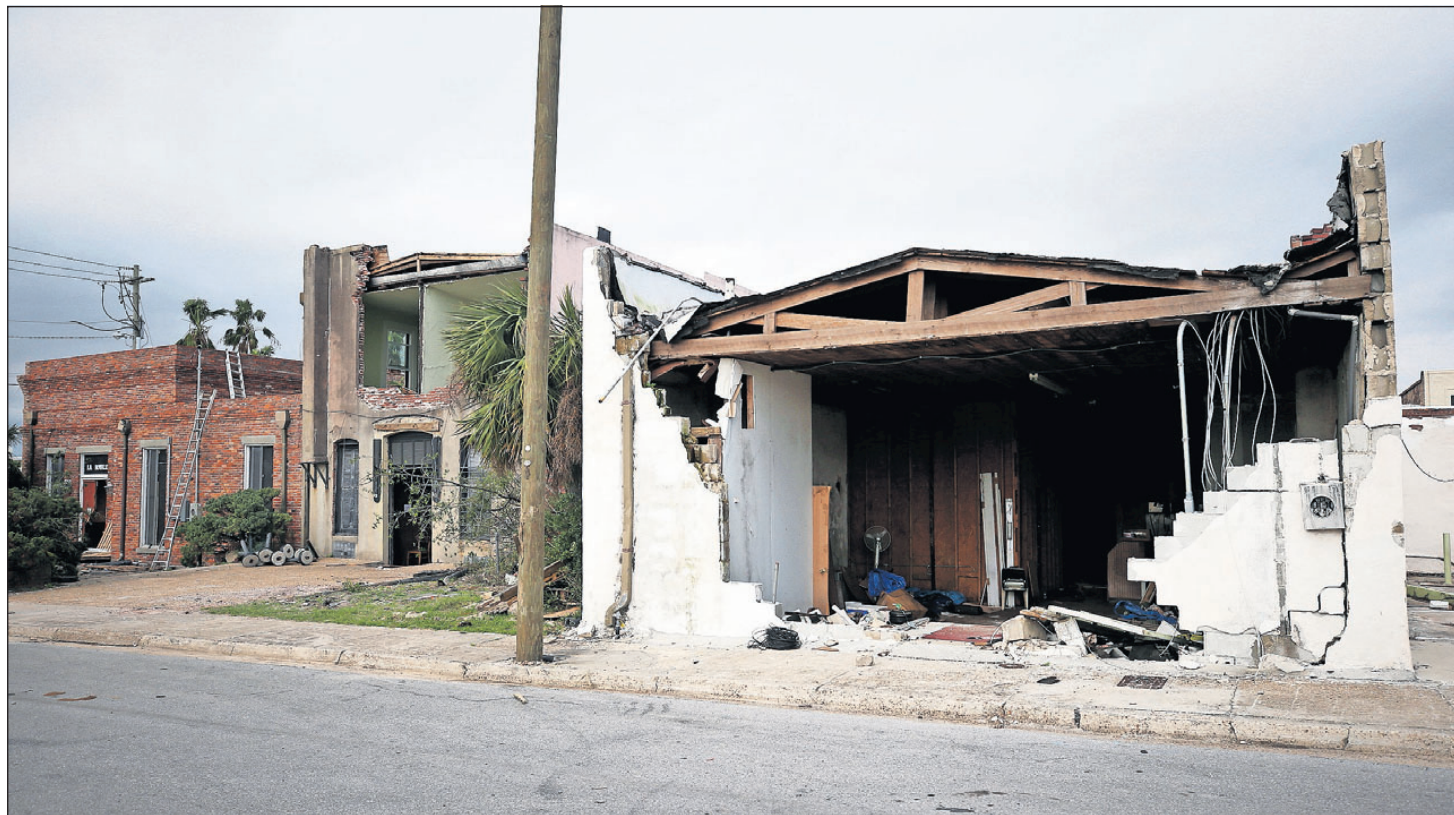
A Downtown Panama City building is missing most of a wall on Tuesday. [PATTI BLAKE/THE NEWS HERALD]
