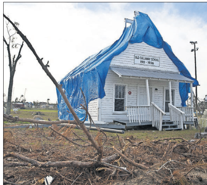
The Old Callaway School House, shown here on Jan. 2, was heavily damaged by Hurricane Michael. [JOSHUA BOUCHER/THE NEWS HERALD]
