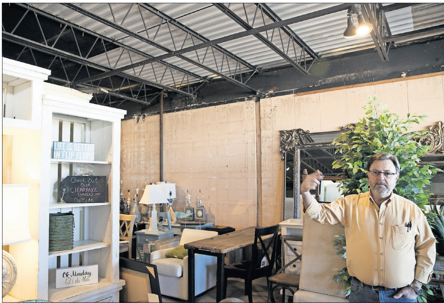
James Johnson, owner of Fowhand Furniture, on Tuesday shows the parts of the building that were damaged by Hurricane Michael. After suffering damage from Michael, the store was able to reopen with some furniture slightly damaged and now heavily discounted.
