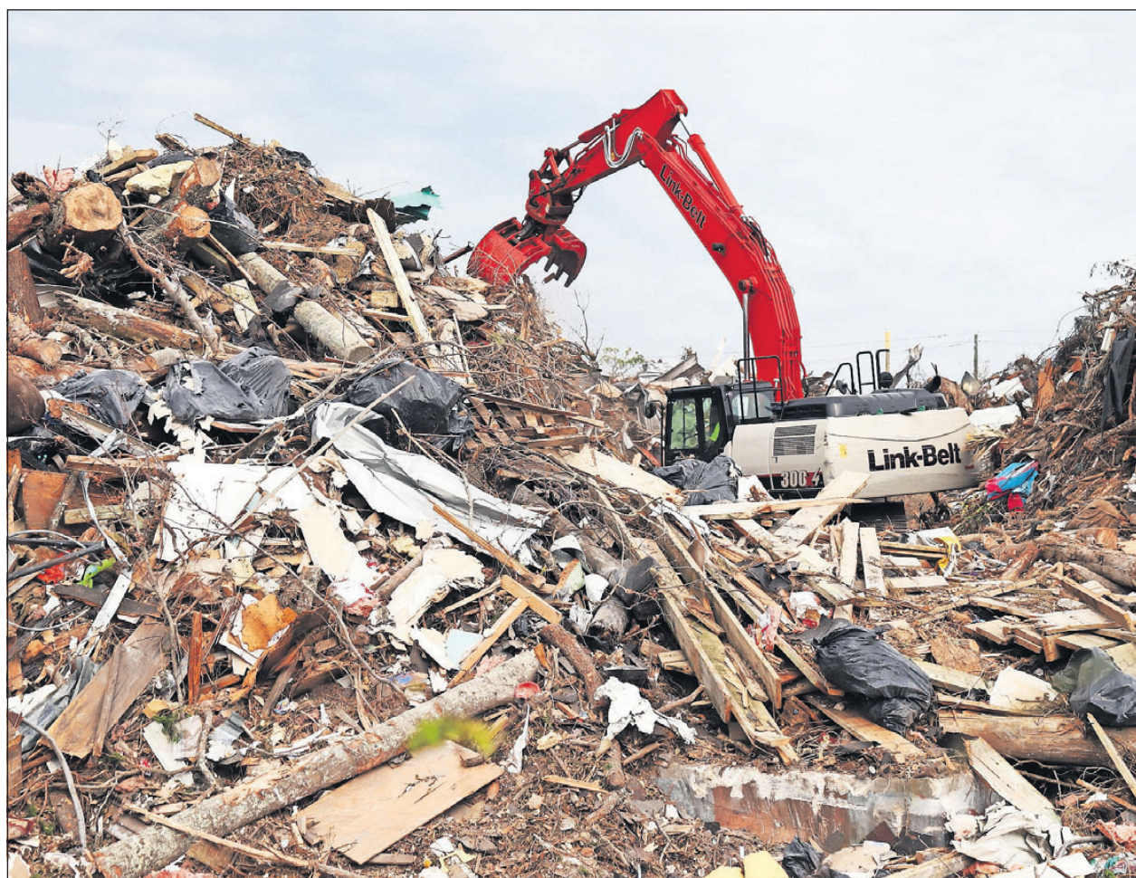
A large excavator moves debris around in a huge pile at a debris-receiving yard on Mulberry Street in Panama City on Thursday. [MICHAEL SNYDER/DAILY NEWS]
