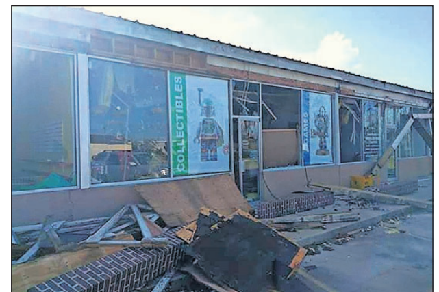
Comic Emporium in Panama City was badly damaged by the storm, then looted on two occasions. [CONTRIBUTED PHOTO]
