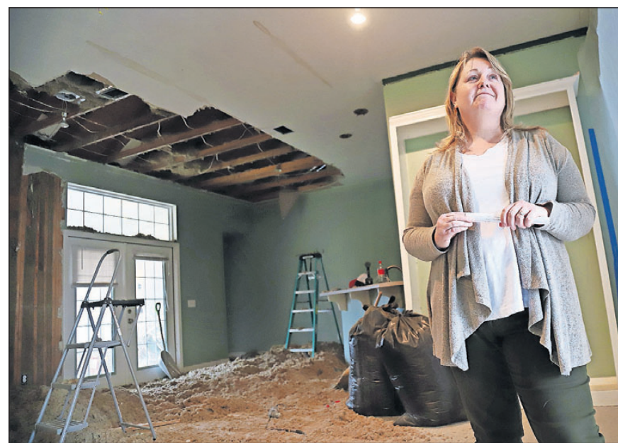
Teacher Lisa Cryderman talks about the work being done on her storm-damaged home in Lynn Haven on Thursday. Her family has been displaced because of the damage. [MICHAEL SNYDER/GATEHOUSE MEDIA FLORIDA]
