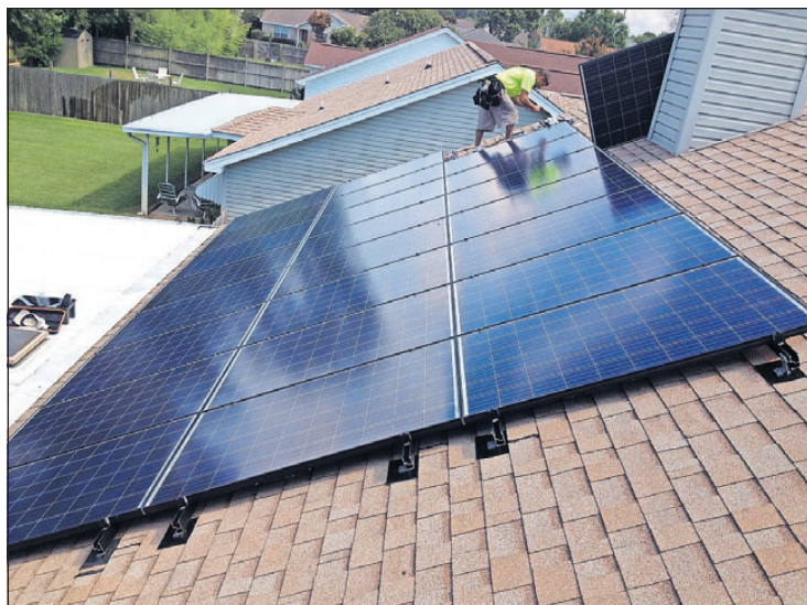
An employee with Pensacola-based Compass Solar installs solar panels on a Gulf Breeze home. The company has expanded its operations into Bay County. [CONTRIBUTED PHOTO]
