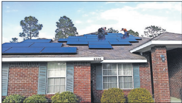
Employee with Pensacola-based Compass Solar install rooftop solar panels on a Milton home. The company has expanded its operations into Bay County.
