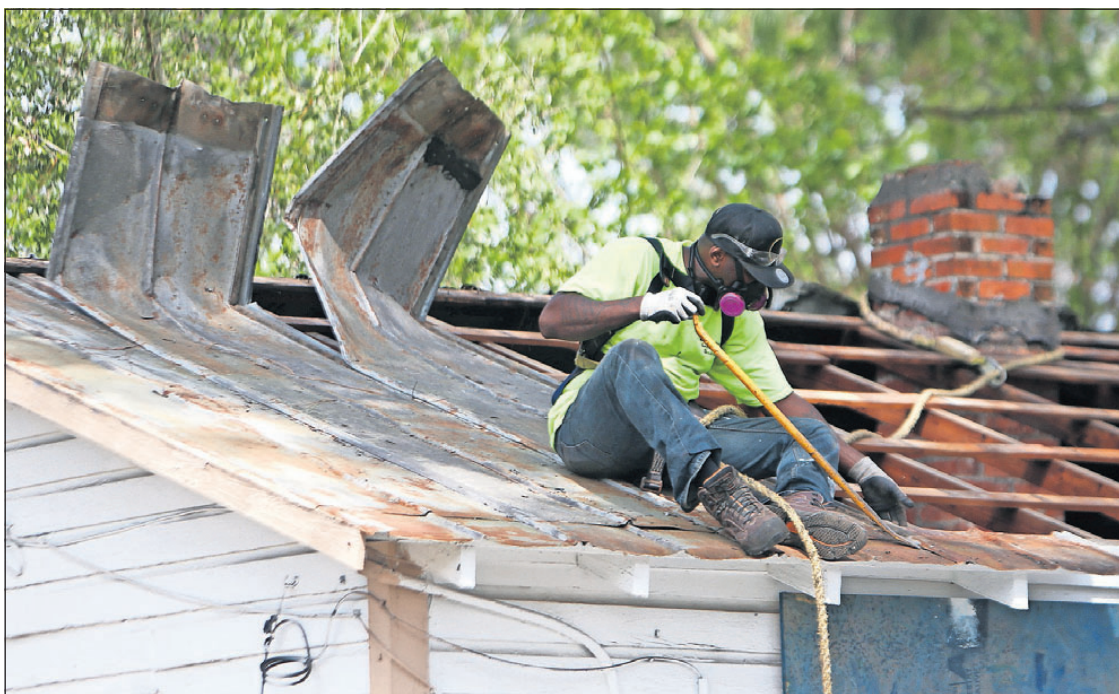
A construction worker removes strips of tin roof from a vacant house Wednesday. Crews are removing the tin roofs from the shotgun houses along Roosevelt, Carver and Washington drives in Panama City after having evicted all the tenants in 2017. [PHOTOS BY PATTI BLAKE/THE NEWS HERALD]
