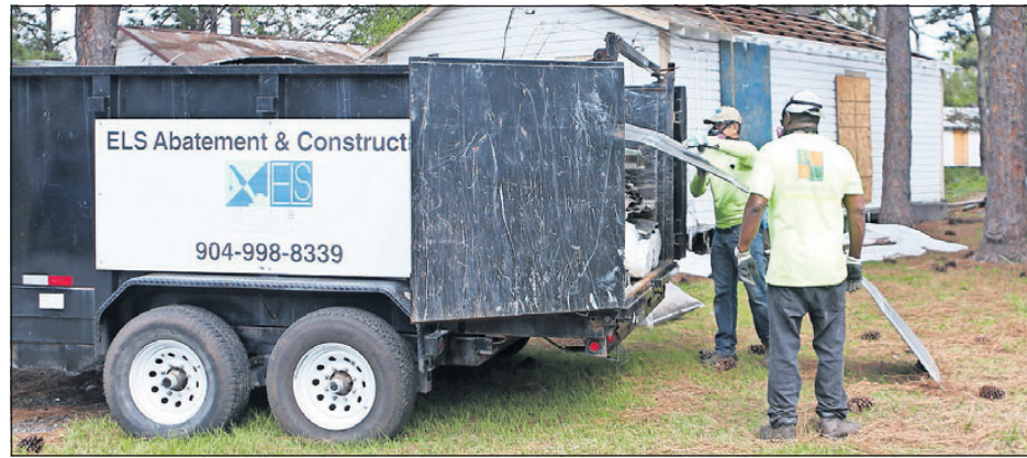
Construction workers load strips removed from a tin roof Wednesday. Demolition of Panama City's shotgun houses is set to begin next week.
