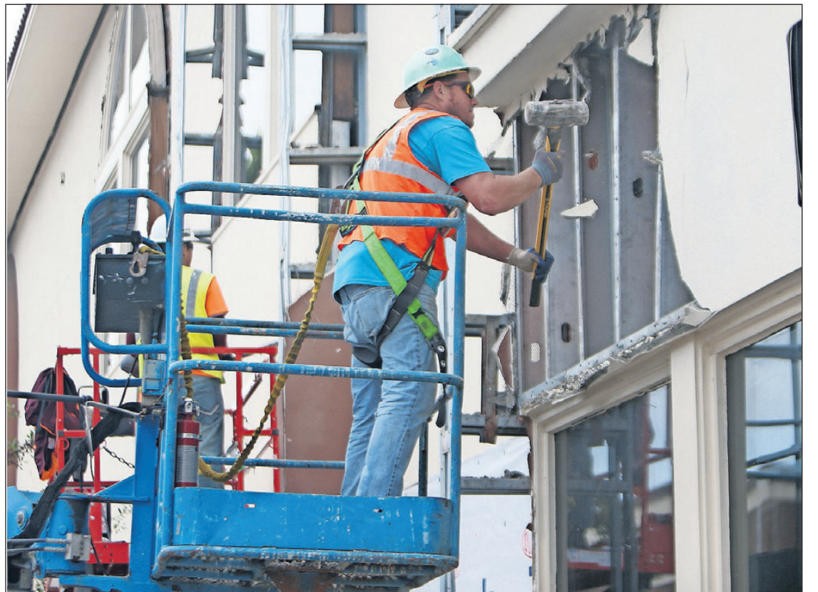
Construction workers remove stucco from the future Panama City City Hall on Thursday. The city had hoped to use the bricks beneath but ultimately will have to construct a new brick wall on the exterior.
