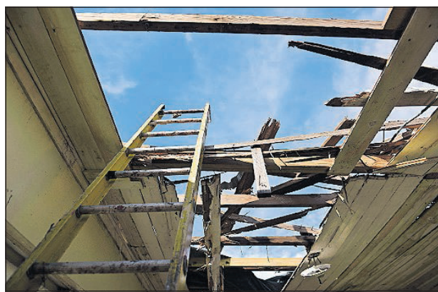
A stairway crosses the hole left by the whip of Hurricane Maria on Nov. 15 in the residence of Edgardo de León, which was declared a total loss by FEMA staff, in Cataño, Puerto Rico. [ASSOCIATED PRESS FILE PHOTO]
