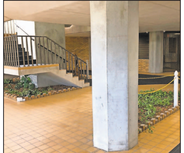
The hallways and stairwells seen here are open to the outside of Building B. The building was completed in 1981.
