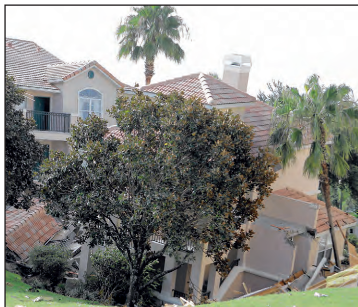
A portion of a building rests in a sinkhole Monday in Clermont, Fla. The sinkhole, 40 to 50 feet in diameter, opened up overnight and damaged three buildings at the Summer Bay Resort.
