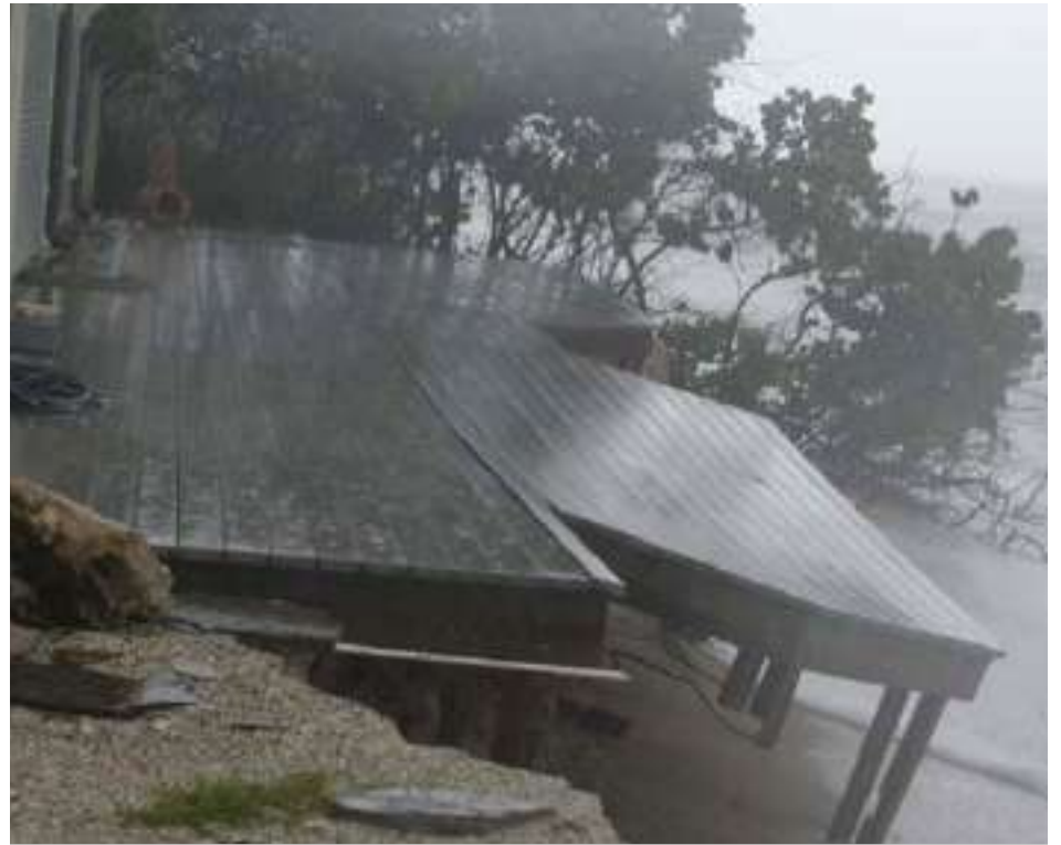
Tropical Storm Andrea did new damage to the property at 2007 Casey Key Road, which suffered erosion during Tropical Storm Debby in 2012 (shown). Image courtesy Sarasota County
